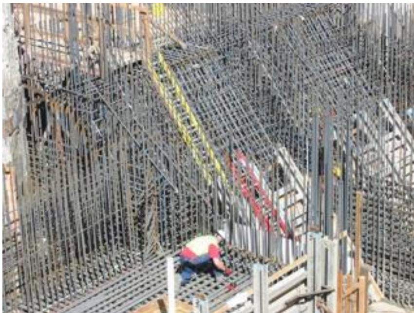
Rebar being set in place for the foundation of a sewage treatment plant pump station. Source: Wikipedia and licensed through Creative Commons.
